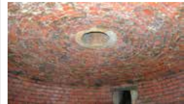
B02 Shallow brick dome to ice-house chamber below floor to game larder
