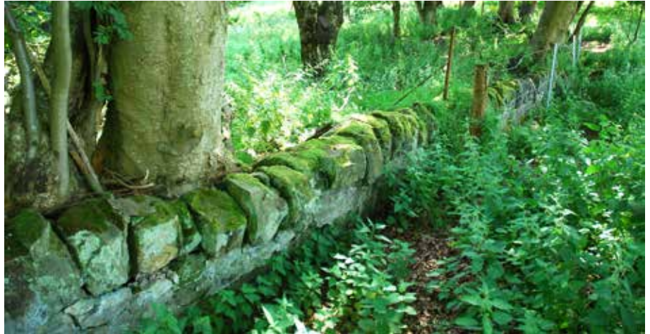
B19 South perimeter wall; section of drystone wall and estate wire fence on south- east flank of Roman hill south- west of house
