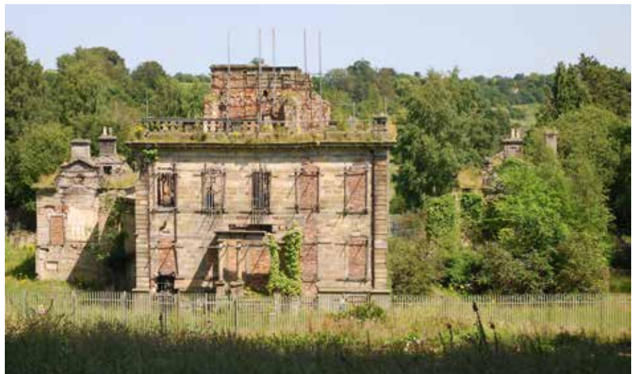
B01 Mavisbank House, west front seen from the lower part of Roman hill
