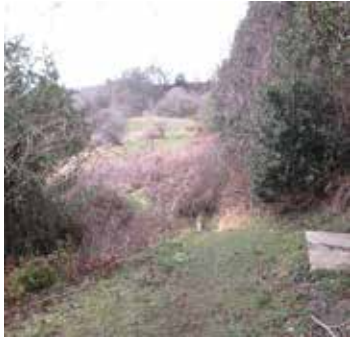
C05 East drive, slumped section near east end
